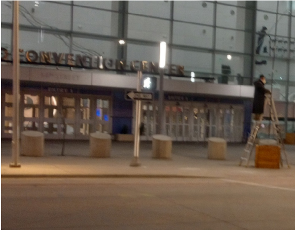
Me attaching a monofilament wire from the side planter to a center planter.
